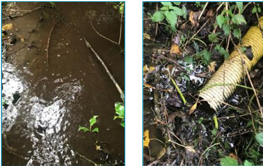
Plate 18.3.8: Silt Deposition and Outfall Pipe
